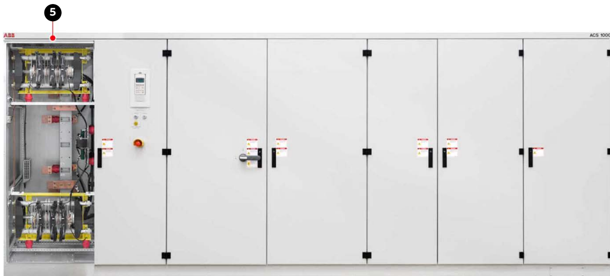
b) ACS1000W with a 24-pulse rectifier
